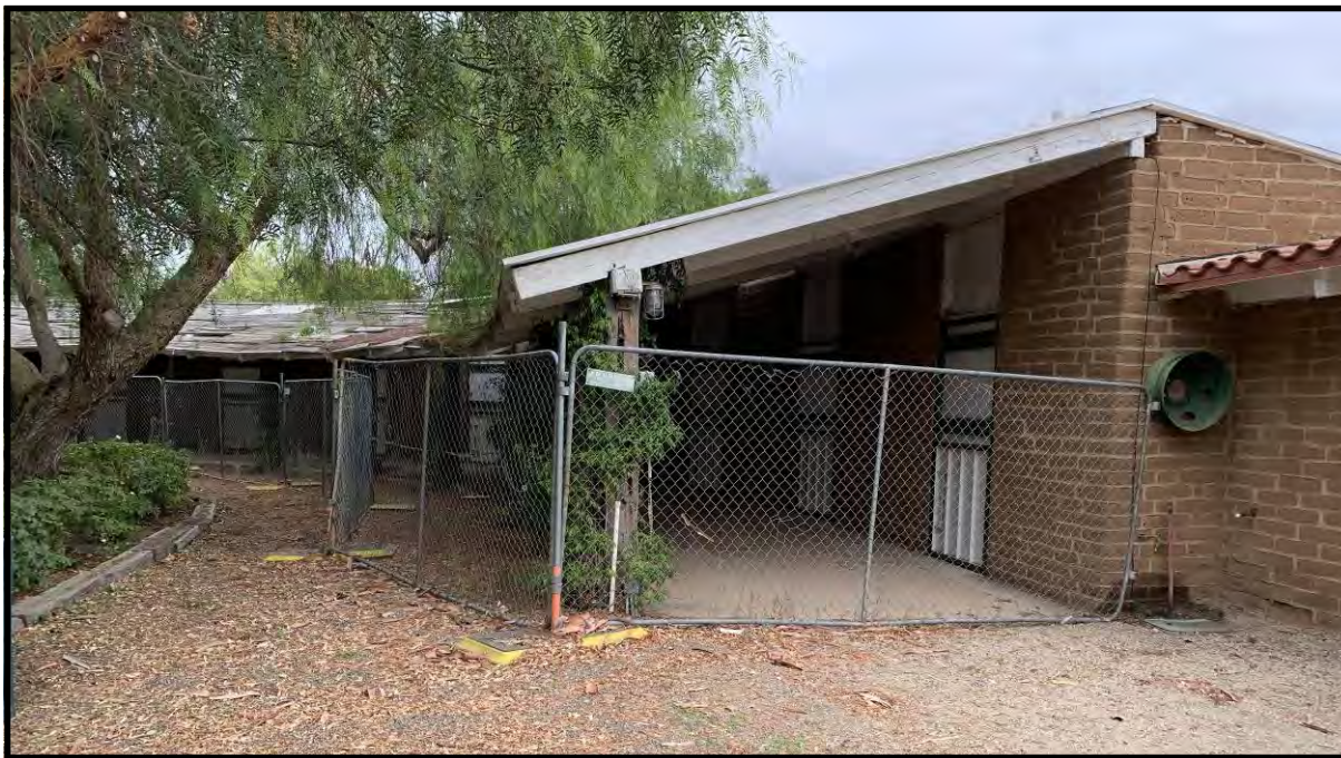
The horseshoe shaped Mare Barn in a dilapidated state. (Photo taken by author on September 28, 2019)
